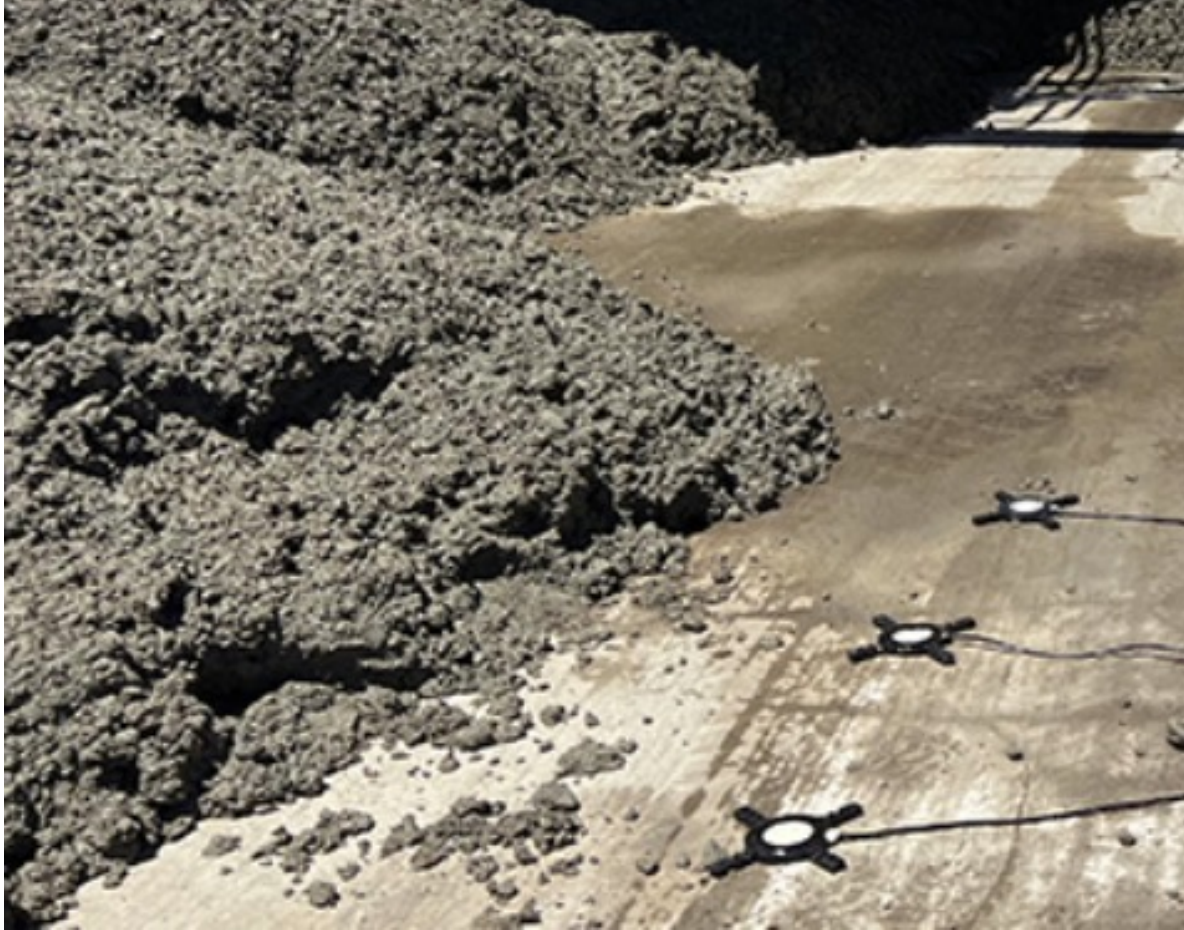
Drop on Roadbed
