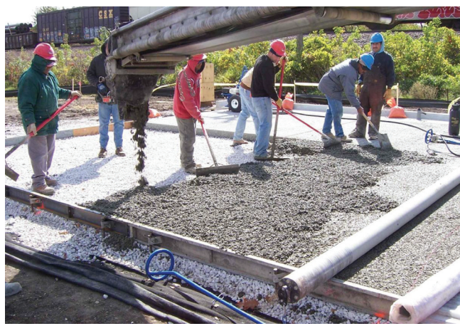
Figure 3.7 Pervious concrete being placed (photo courtesy of John Kevern, University of Missouri-Kansas City)
