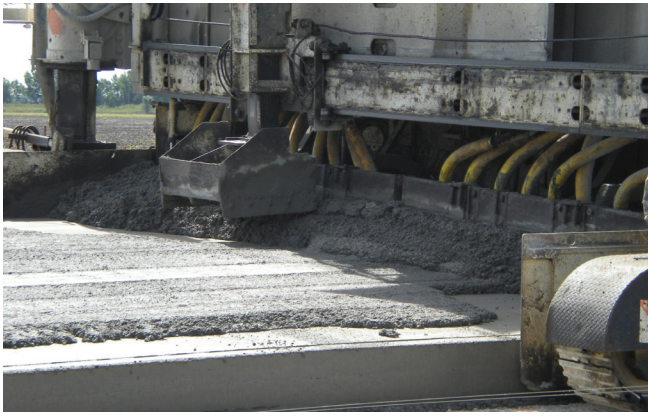
Figure 5.12 Top lift being placed on the bottom lift (photo courtesy of Gary Fick, Trinity Construction Management, Inc.)
