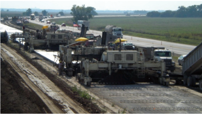
Figure 5.13 Two-lift paving on I-70 in Kansas (photo courtesy of Gary Fick, Trinity Construction Management, Inc.)
