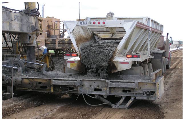
Figure 5.7 Tractor trailer concrete hauling unit (photo courtesy of Gary Fick, Trinity Construction Management, Inc.)
