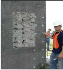
50 kHz UPV transducers with 1 ft grid direct test patterns from North-South and East-West
