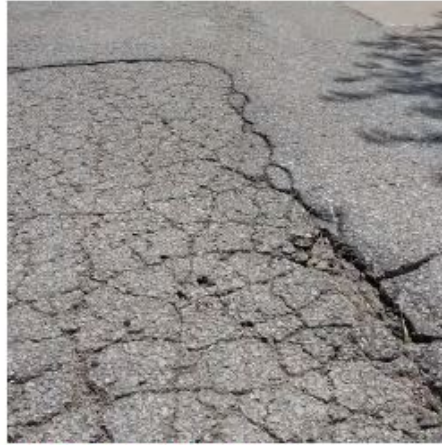
Figure 10b. High-severity alligator cracking
