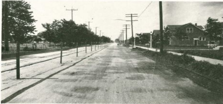
Condition of the old pavement before work of renewing the surface with a layer of concrete was started. The shadow of the barricade on the left shows how the old pavement was worn into waves by traffic.
