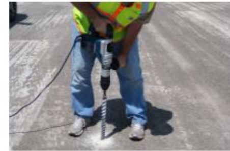
Figure 6. Hammer drilling to check pavement thickness (Photo courtesy of David White, Iowa State University)
