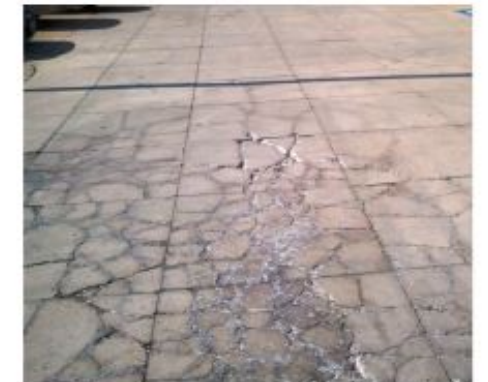
Figure 8. Failure of concrete overlay sections in locations where the existing asphalt pavement surface was entirely removed through milling because of lack of core information
