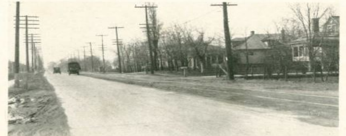
South Seventh Street Road, Terre Haute, Ind., showing condition of concrete resurfacing after 8 years' service.
