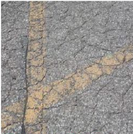
Figure 10a. Low- to medium-severity alligator cracking
