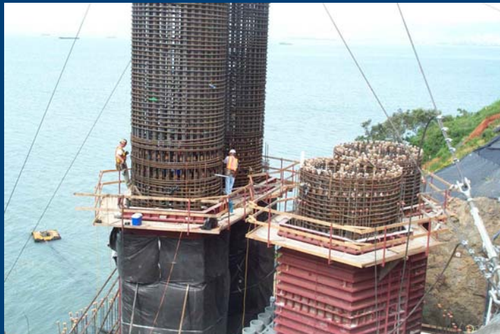
Piers for the San Francisco-Oakland Bay Bridge, courtesy of John Gajda, CTLGroup
