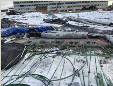
Inadequate protection caused blowout
