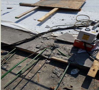
PT Blowout due to cold concrete
