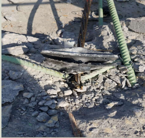
PT Blowout due to cold concrete
