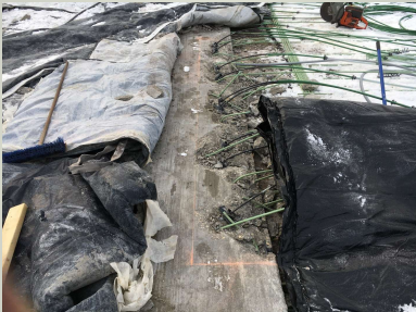
PT Blowout due to cold concrete
