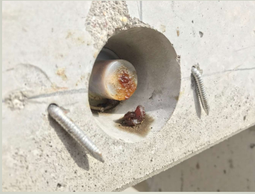
Leaking cap, needs replaced
