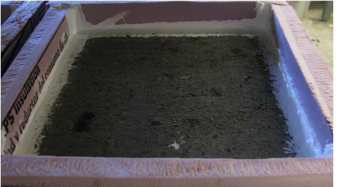
Photo 4: Showing scaling of ASTM C672 panel #4 after 50 cycles.
