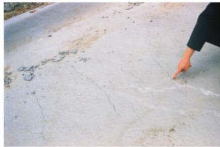
FIGURE 18-7. Typical plastic shrinkage cracks.
