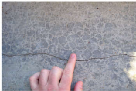
FIGURE 18-6. Crazing cracks are a network of fine cracks shown, compared to a drying shrinkage stress crack.
