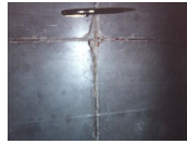
Spalled joints in 1-year old facility
