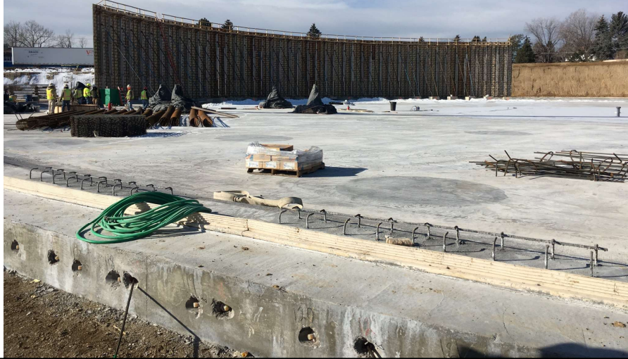
Denver Water Hill Crest – Three 15 million gallon tanks
