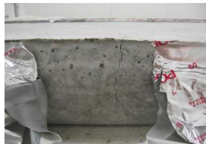
IC 0.30 Concrete 0.4 mm wide crack observed @ 43 days
