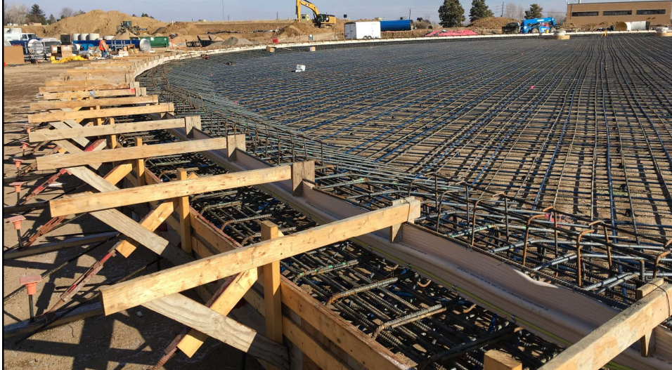
Denver Water Hill Crest – Three 15 million gallon tanks
