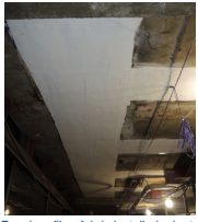
FRP carbon fiber fabric installed prior to PT work to avoid overstressing the structure during detensioning/retensioning
