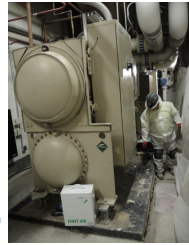
Existing Mechanical Room: >>> Protection of equipment from dust and debris produced by demolition of slab to be constructed
