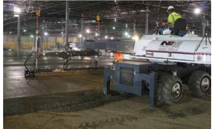
Fig 6: Placement of the slab-on-ground floor for the Target store in Inver Grove Heights, MN, on January 31, 2012
